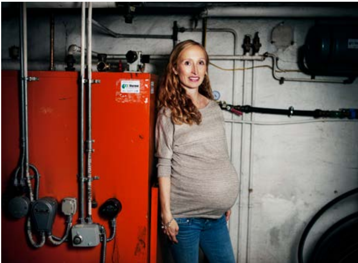
CLEANER ENERGY: By replacing the oil burner, Nina Merete Wiley makes sure her coming twins can breathe cleaner air. (Photo: Therese Alice Sanne/VG /NTB Scanpix).
